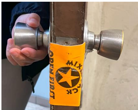
Figure 18: Picture of Tape on the Door
